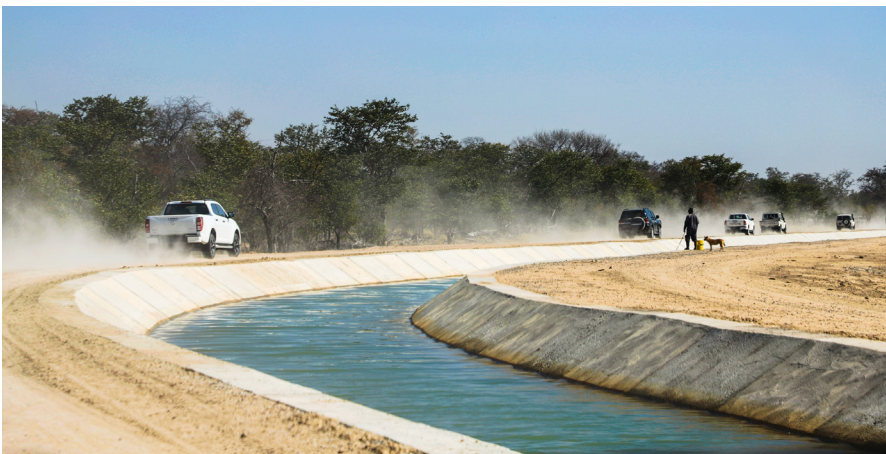
A drought relief project undertaken by Power Construction Corporation of China in Cunene Province of Angola on September 7, 2023 (XINHUA)
