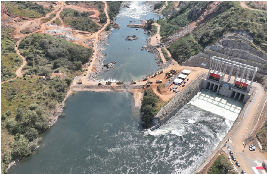
This aerial photo taken on May 20, 2023 shows a ceremony for the temporary diversion of the Cuanza River at the site of the Chinese-built Caculo-Cabaca Hydropower Station in Cuanza Norte province, Angola. (XINHUA)
